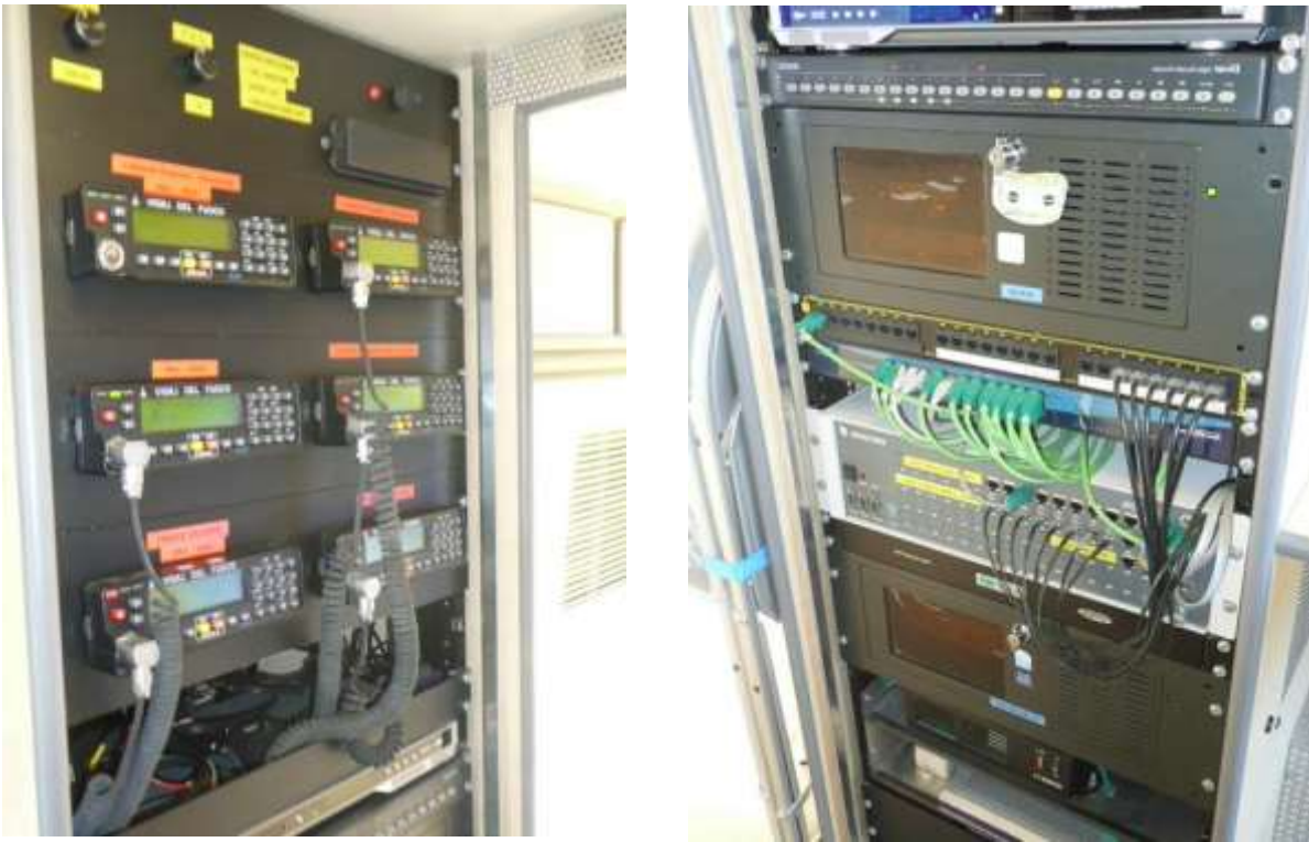
Figure 11 ICT equipment: radio links and servers
