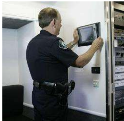
Figure 16 Touch control panel
