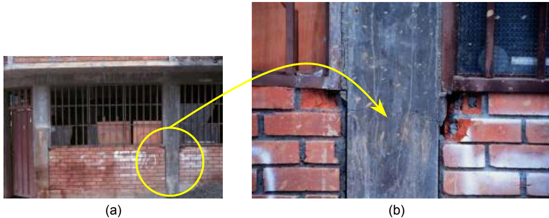
Fig. 4-22 (a) A Colombian self-built RC structure, featuring “short” columns; (b) Close-up of a short column (adjacent to two mid-height infill walls) that failed in shear. (source: Taucer, 1999)
