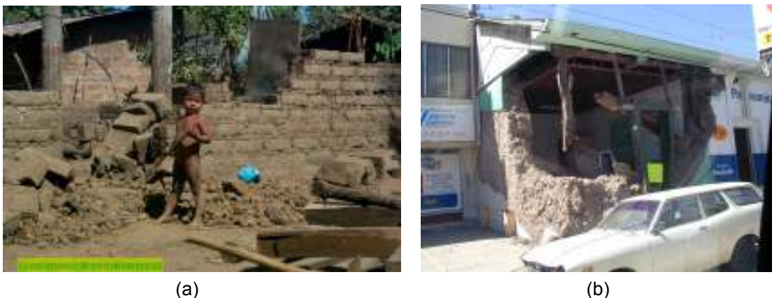
Fig. 4-33 (a) Collapsed adobe house in Canto La Concordia, near Jiquilisco [source: Salvadorean Programme for Research on Development and Environment (PRISMA)]; (b) Near-collapse of an older adobe structure in Santa Tecla. (source: photo by Conrad Paulson and Larry Hultengren – annotated picture from EERI special newsletter report on the El Salvador earthquakes of 13 January and 13 February, 2001)
