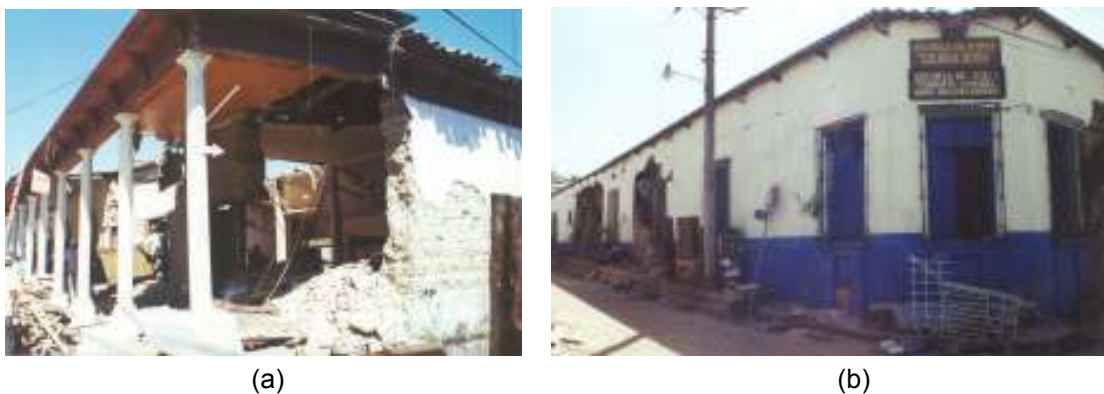
Fig. 4-39 (a) Destruction of an adobe portal in Cojutepeque; (b) A severely damaged adobe school in Cojutepeque where some students were killed. (source: photo by Manuel López Menjivar, University of El Salvador – annotated picture from EERI special newsletter report on the El Salvador earthquakes of 13 January and 13 February, 2001)
