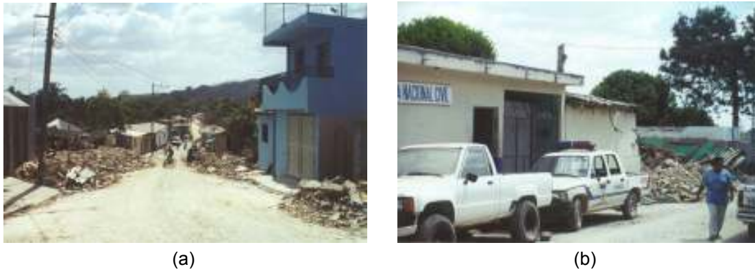
Fig. 4-46 (a) Mixto construction in the town of Santa Cruz Analquito still standing, but surrounding a destroyed adobe construction; (b) House of mixto construction in Santa Cruz Analquito still standing next to an adobe house turned into rubble. (source: photo by Manuel López Menjívar, University of El Salvador – annotated picture from EERI special newsletter report on the El Salvador earthquakes of 13 January and 13 February, 2001)
