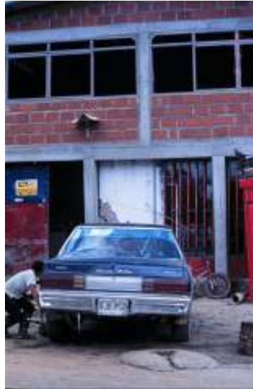
Fig. 4-23 Lack of vertical continuity of columns in a Colombian self-built RC structure.
