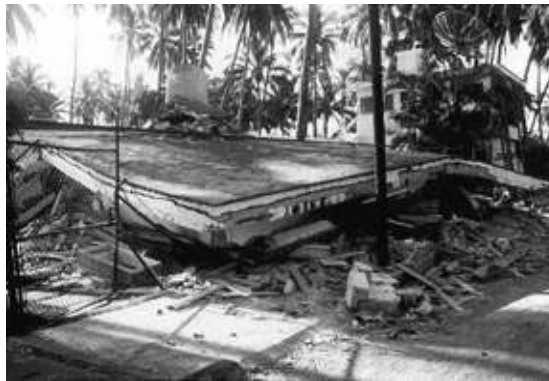
Fig. 4-25 This two-story home in Manzanillo collapsed due to a heavy roof and inadequate walls. (source: EERI, 1995)
