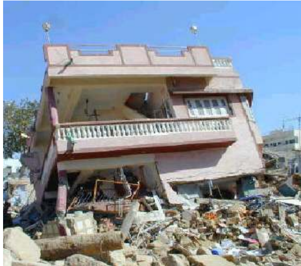
Fig. 4-51 Typical soft storey and torsion collapse in Bhuj. (source: Gujarat Relief Engineering Advice Team - GREAT, 2001)
