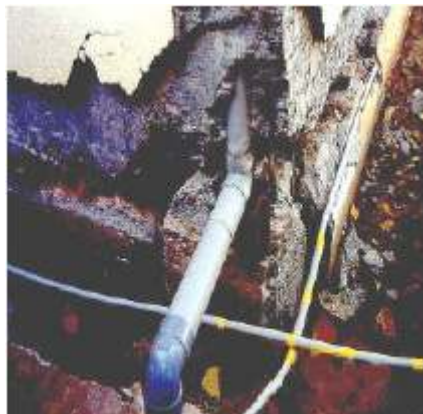
Fig. 4-53 Separation between the ground beam and the column junction caused by crushing of the concrete (city of Sukhpur). The damage worsened by the presence of a plastic pipe within the column. (source: Gujarat Relief Engineering Advice Team - GREAT, 2001)
