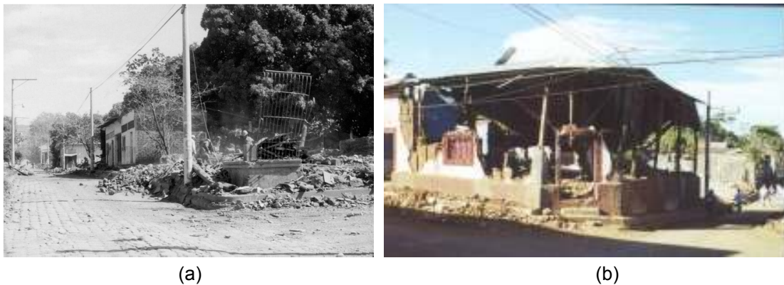
Fig. 4-32 (a) Collapsed adobe house in San Agustín, of which only the door remains standing after the 13 January earthquake; behind are houses of mixto and lámina , which have survived the earthquake (source: Bommer et al., 2002); (b) Damaged adobe house in Santiago de María. (source: photo by Julian Bommer – annotated picture from EERI special newsletter report on the El Salvador earthquakes of 13 January and 13 February, 2001)
