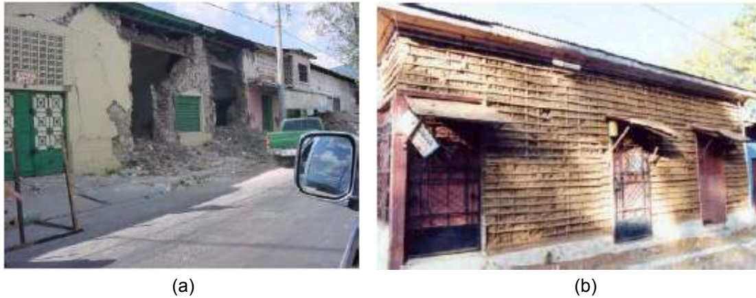
Fig. 4-31 (a) Typical adobe house damaged by the earthquake; (b) Bahareque structure, which suffered mud cover spalling. (source: JSCE, 2001)
