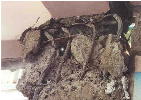
Fig. 4-52 Heavy compressive stresses and large deformations caused total destruction of the column head; heavily bent longitudinal reinforcement is shown. The large spacing of stirrups did not provide effective confinement of the concrete core. (source: Gujarat Relief Engineering Advice Team - GREAT, 2001)
