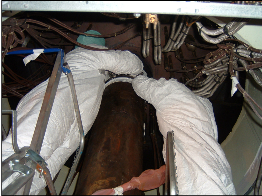
Figure 5. Example of robot installation for automated UT on the pressurizer surge line
