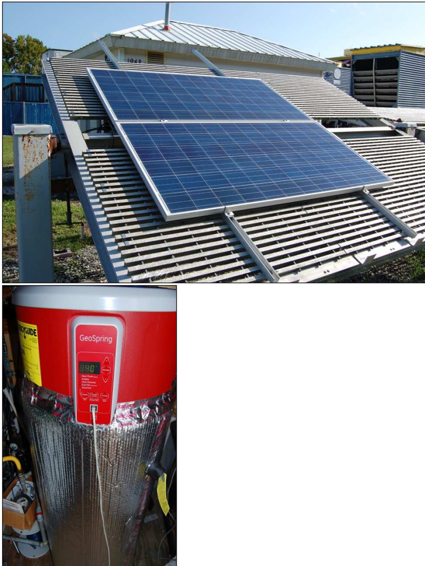
Figure 1: PV modules (310 Watts each) and 189–Liter HPWH shown with added insulation
