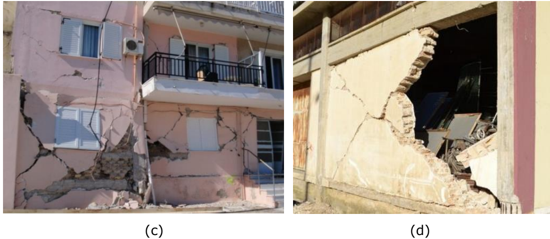
Figure 2.5 Example of damage to masonry infills in RC multi-storey buildings: (a)-(b): L'Aquila 2008, M_s 6.3; Source [21]; (c)-(d) Kefalonia 2014, M_s 5.9; Source [22].
