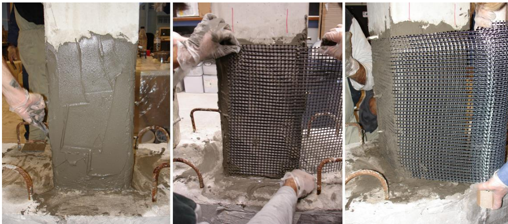
Figure 3.7 Seismic retrofitting procedure of RC column base via TRM jacketing to increase its deformation capacity: (a) Application of first mortar layer; (b)-(c) application of the textile into the mortar to complete TRM jacketing; Source [49].
