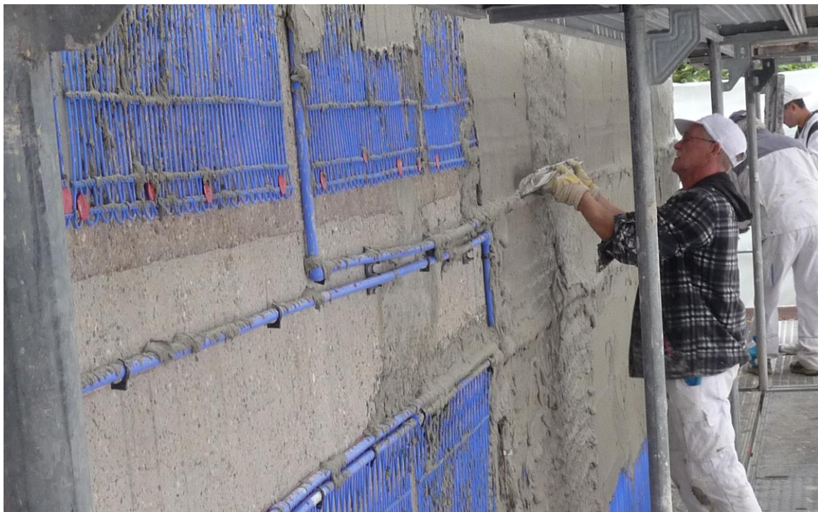
Figure 3.22 Surface heating under thermal insulation is being installed on an exterior wall for the first time as part of a renovation project, whereby the capillary tube mats (pictured) are applied to the concrete facade and then plastered over with adhesive mortar. © IZES gGmbH.
