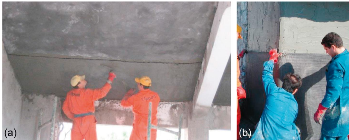
Figure 3.13 Strengthening of (a) concrete slabs and (b) stone masonry walls in a mixed concrete–masonry school building. Kind permission of Triantafillou (2007); Source [57].
