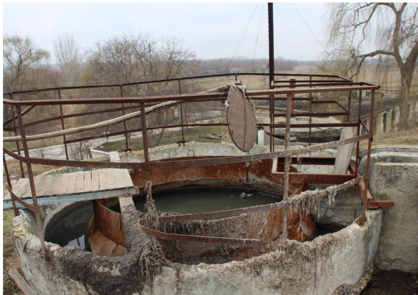
Figure 17 - The WWTP of Leova: primary (mechanical) treatment stage. Courtesy P.Panus.
