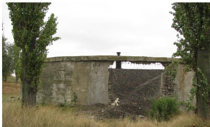
Figure 16: Damaged Biological filter, Cahul. Source: P.Panus.
