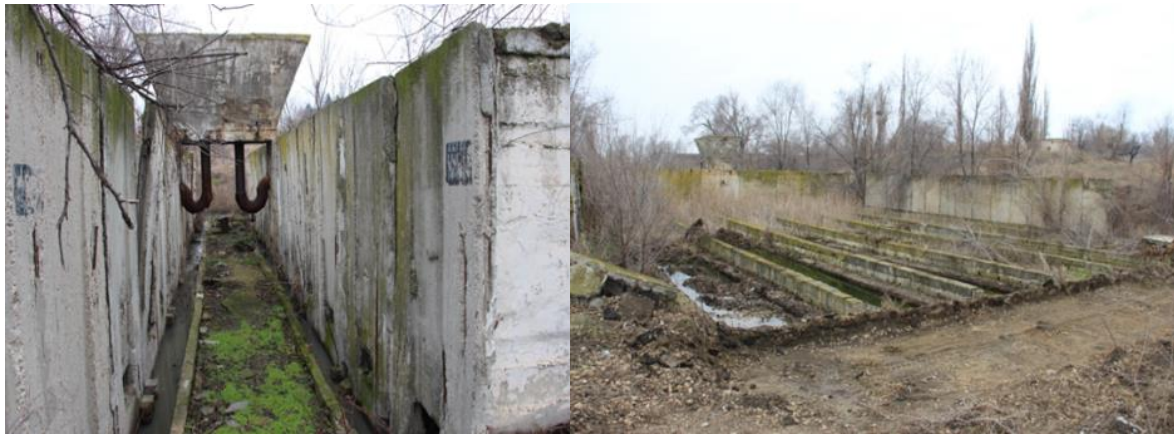
Figure 18 - Biological filters in the WWTP of Cantemir. Courtesy P.Panus.
