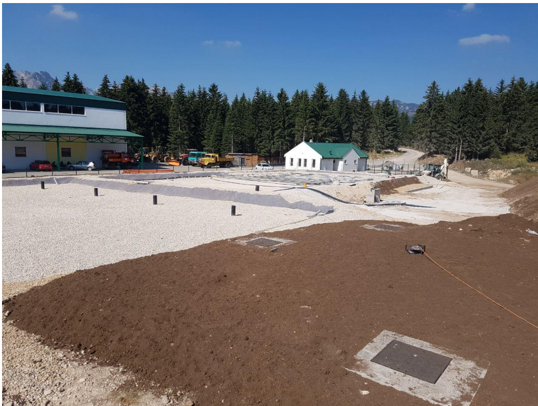
Figure 22 – Žabljak: realization of a constructed wetland for sludge treatment, next to the waste recycling centre (courtesy Gregor Plestenjak)
