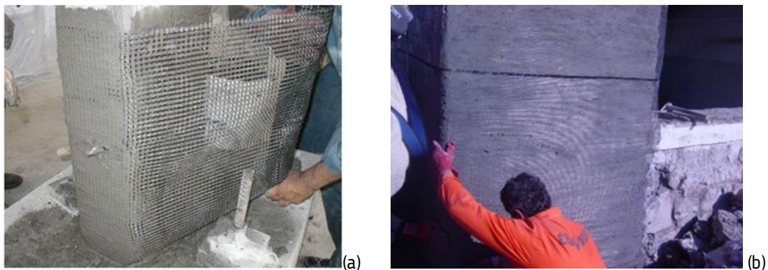
Figure 13. Applications of TRM jacketing on (a) RC column and (b) masonry wall
