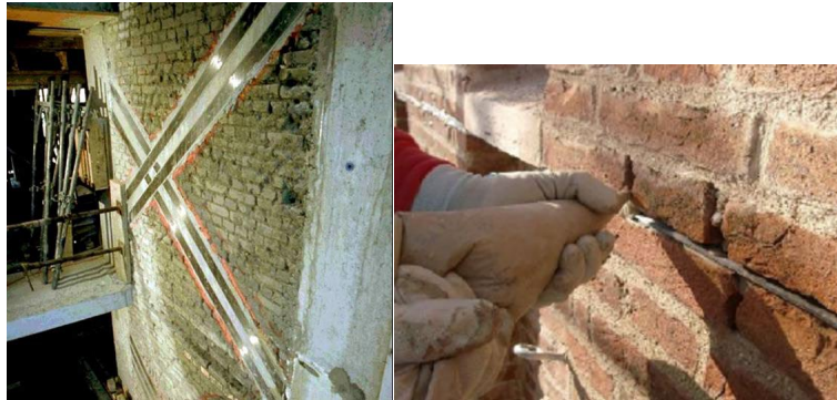
Figure 12. FRP retrofitting of masonry: (a) In-plane shear strengthening with diagonal and possibly vertical/horizontal strips; (b) near-surface mounted FRP strips;
