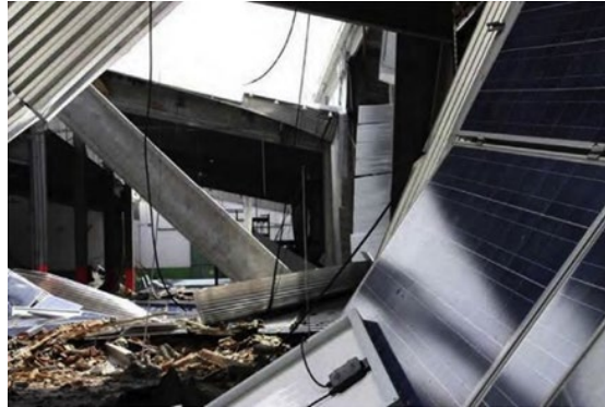
Figure 8. Collapse of an RC building, which received only energy retrofitting after the 2012 Emilia-Romagna earthquake.
