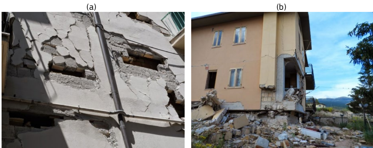
Figure 2. Seismic damage after the 2009 L'Aquila earthquake (a) Damaged infills in RC frame structure; (b) Soft-storey failure.
