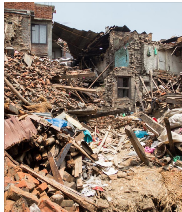
Earthquake damage The 2015 earthquake in Kathmandu caused severe damage to buildings, not only in the Kathmandu metropolitan area, but also in the surrounding towns and villages. © World Travel Photos - stock.adobe.com
