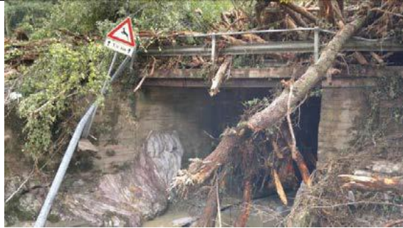
High single arch bridge but with a small width, not enough to allow intense transport of large woods
