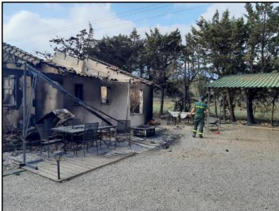
Figure 24. Examples of fire damage (campsite and house destroyed).
