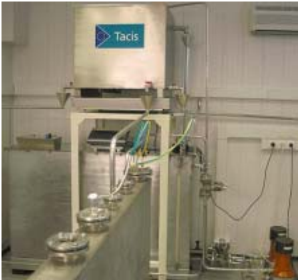
Training Room in ULBA showing tanks similar as to those installed in the facility
