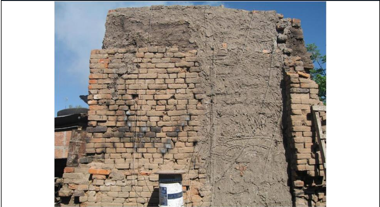
Figure 15: Detail Salamanca 2, stationary kiln using steam-injected Combustóleo
