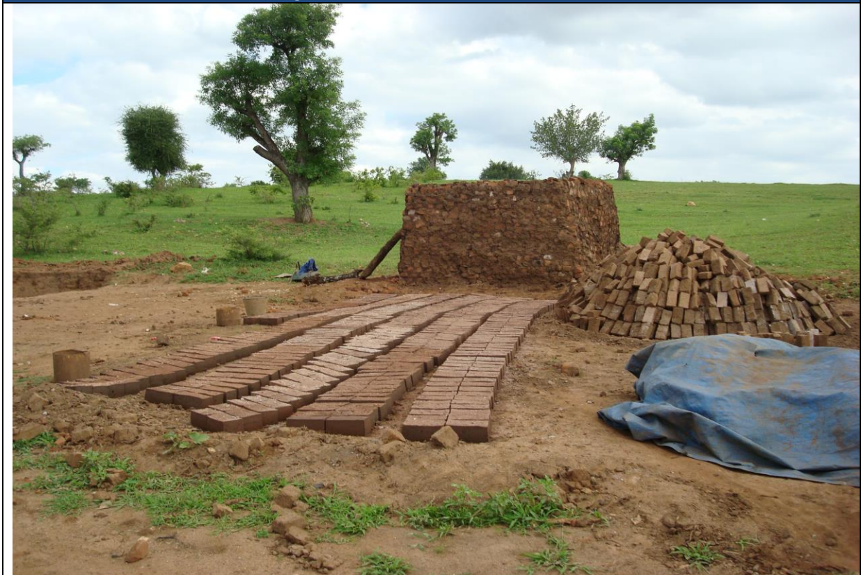
Wet bricks laid out to dry, with PVC tarpaulin to cover against rain. Clay is mined from a quarry to the left.
