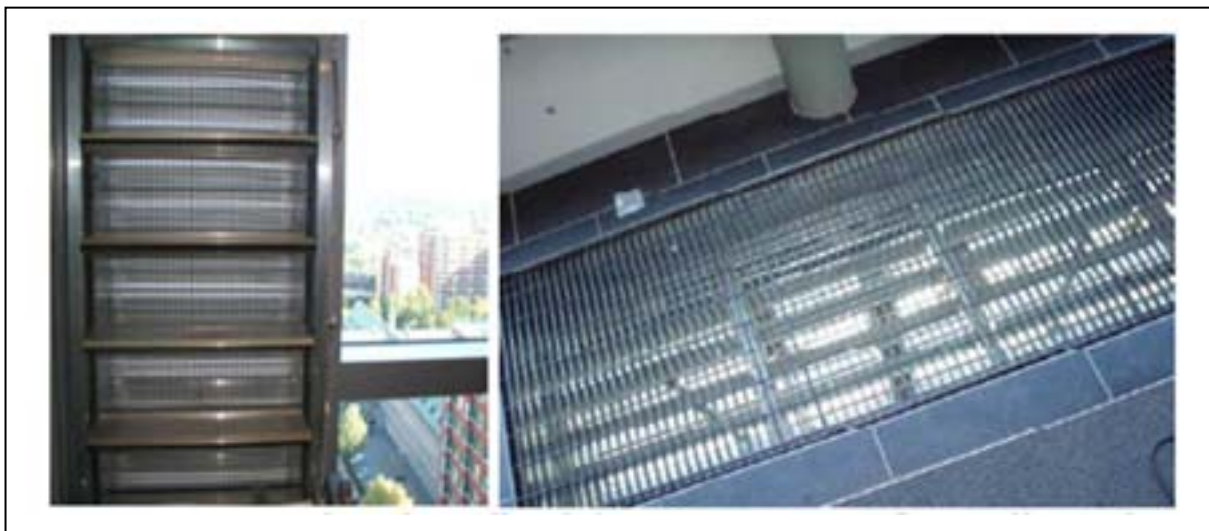
An example of corridor inlet vents (left) and atria connecting floor vents (right), installed for natural ventilation of the Concordia University building in Montreal (Canada)
