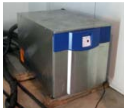
Fig. 2. Rotartica Solar 045 absorption chiller
