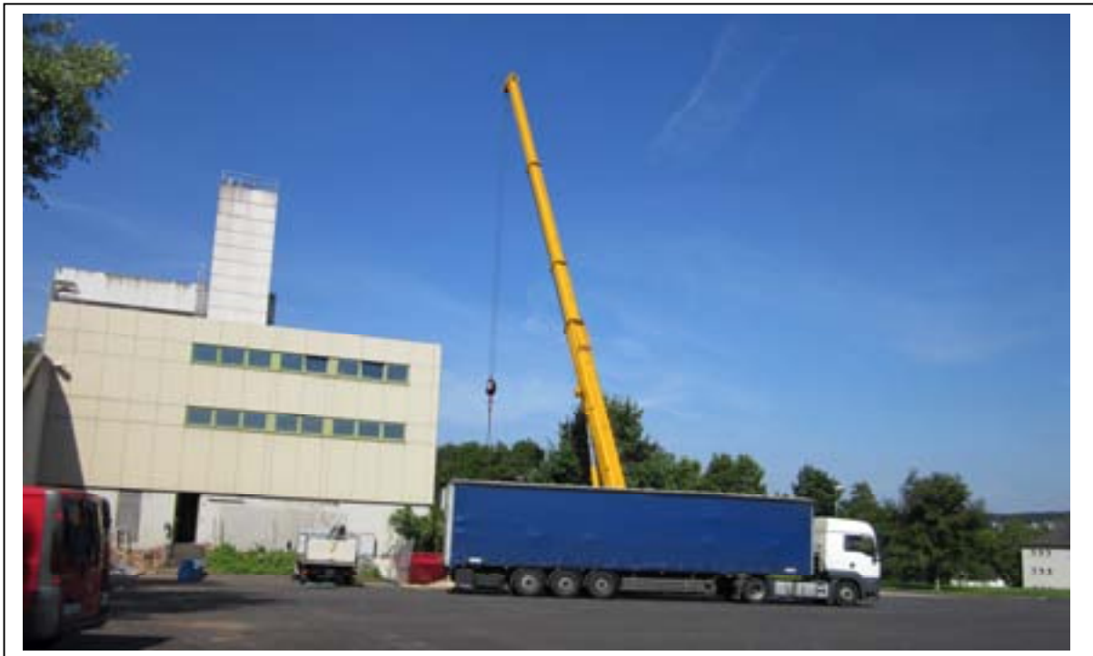
Installation of the new woodchip-fired boiler into the boiler house (source: JCI)
