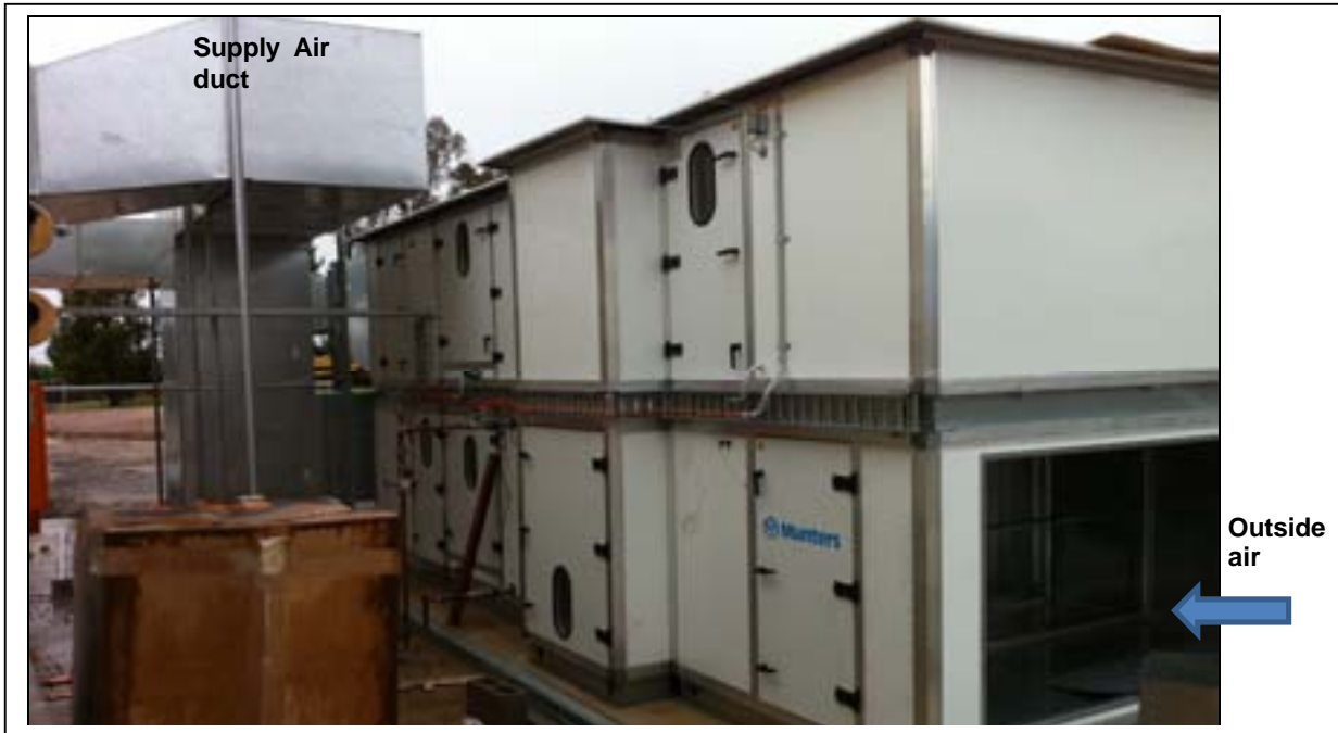
Figure 14: Two stage evaporative cooler – installed
