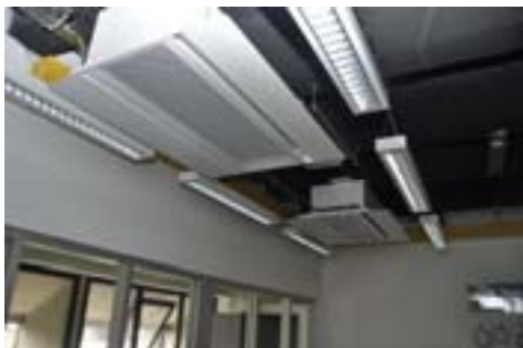
Figure 3. Active Chilled Beam – Indoor Environmental Quality Laboratory.
