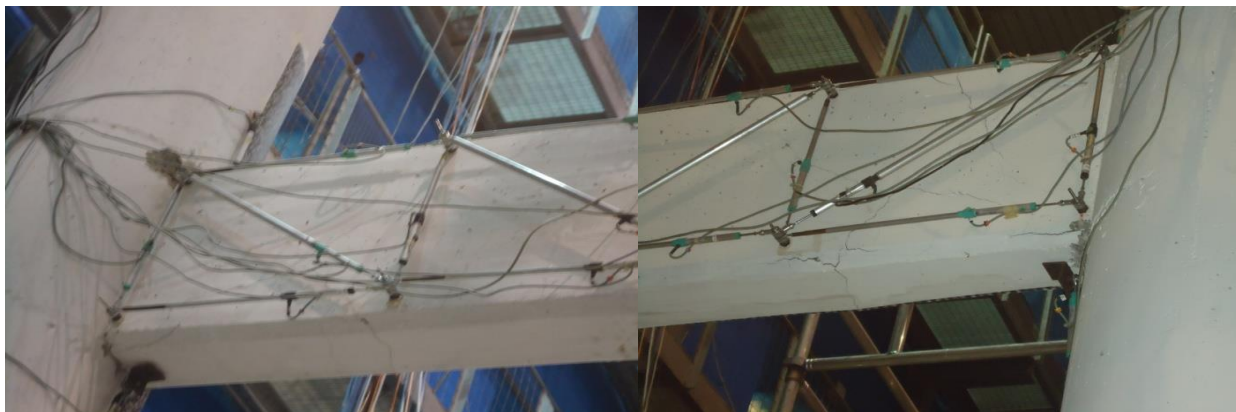
Fig. 10.18 Shear cracks pattern in the transverse beam of pier 11 after test k09
