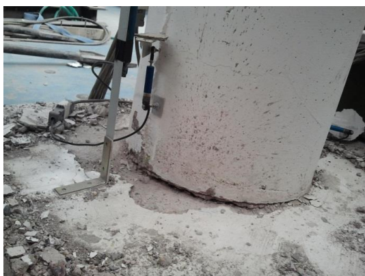
Figure 6.10 Crack opening for bar slippage
