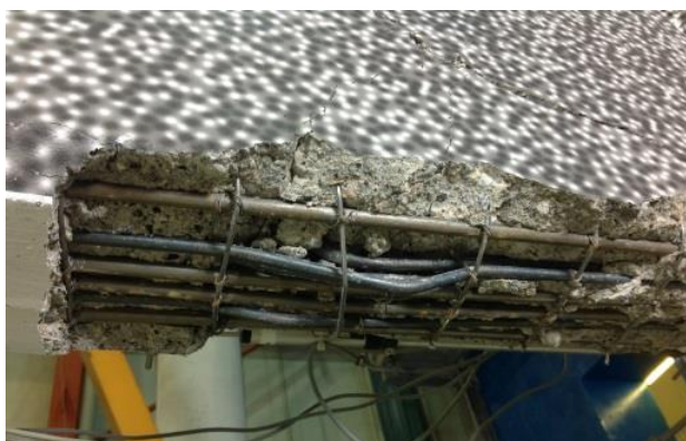
Fig. 10.28 Blow up of the transverse beam damage on short pier after test k12
