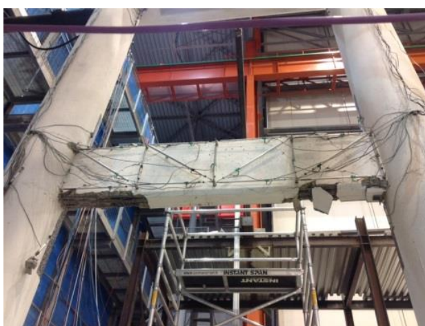
Fig. 10.26 Transverse beam damage on pier 11 after test k12
