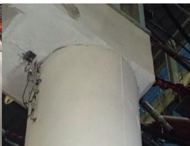
Fig. 10.27 Crack opening at the top of a column in the Short pier after test k12
